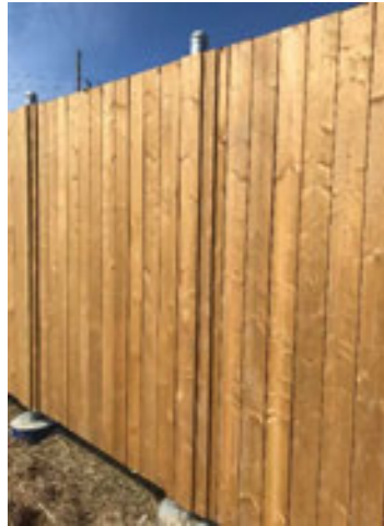
Figure 6-1: Existing wooden barrier installed on the corner of Montreal Street and John Counter Blvd.
