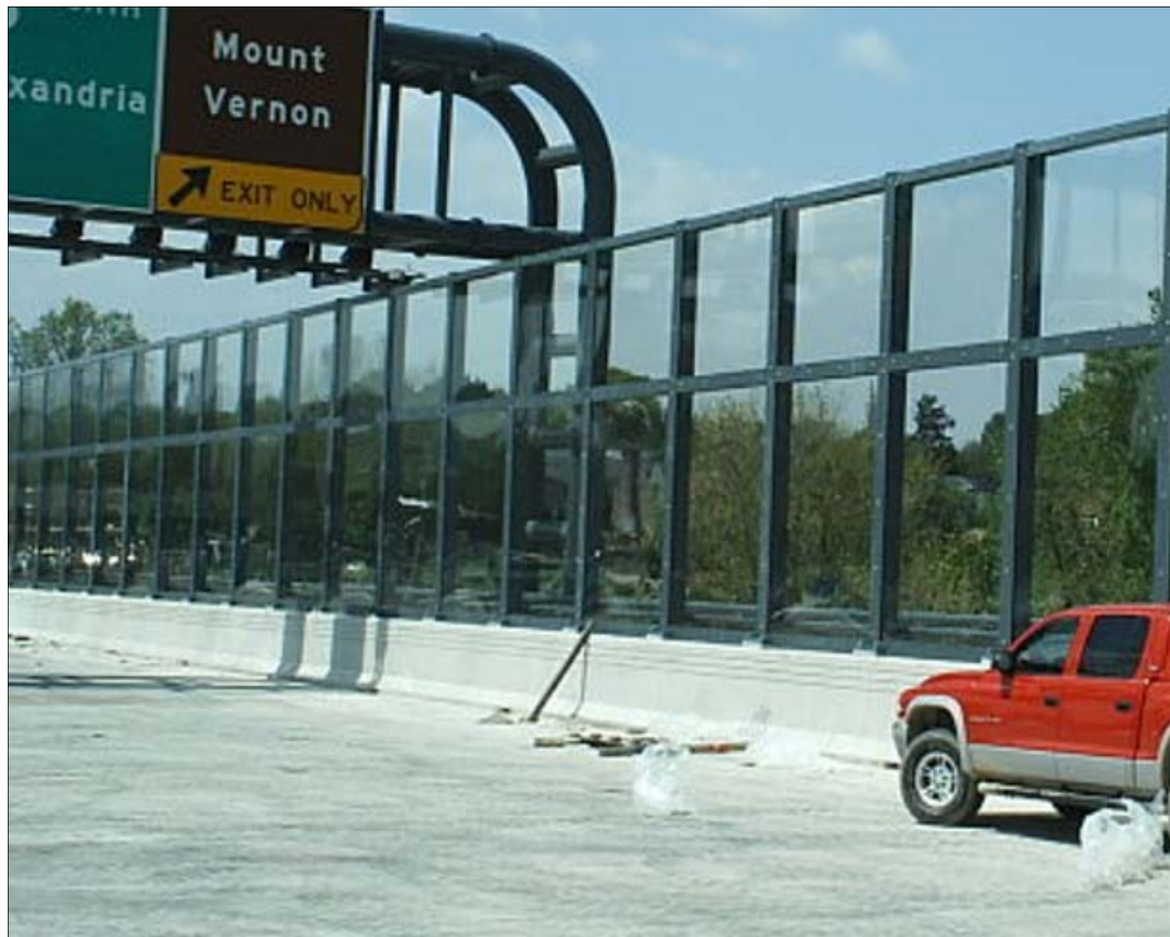
Figure 6-3: Example of a permanent noise barrier installation on a pre-existing traffic crash barrier. NBRE09-2 would follow a similar set-up
